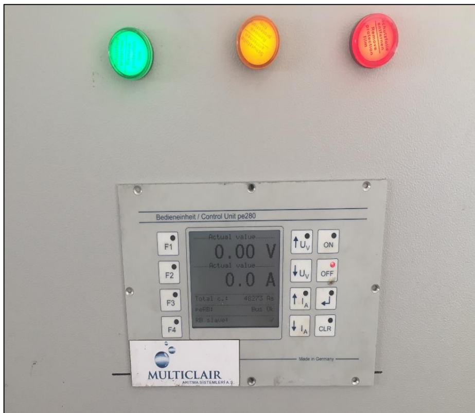
Figure 3.5. E&E process reactor control panel.
