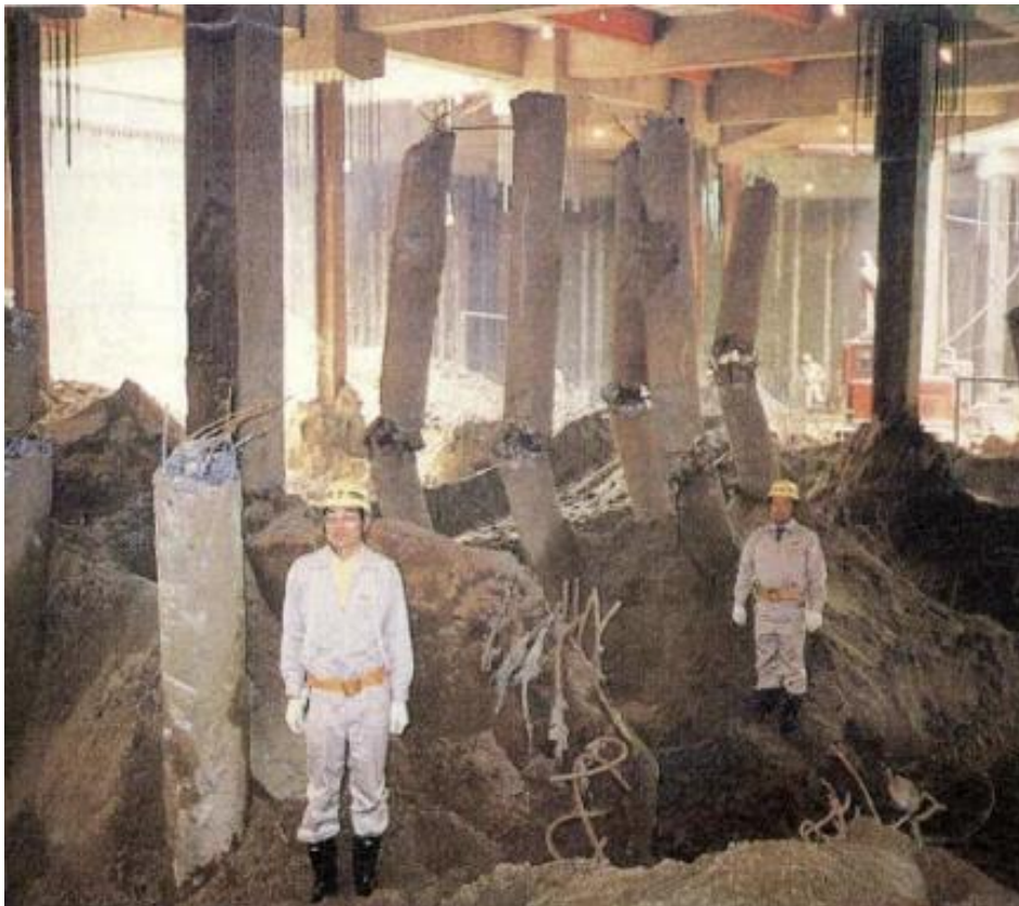
Figure 2.3. Damaged piles under NHK building after Niigata earthquake (Hamada, 1991)
