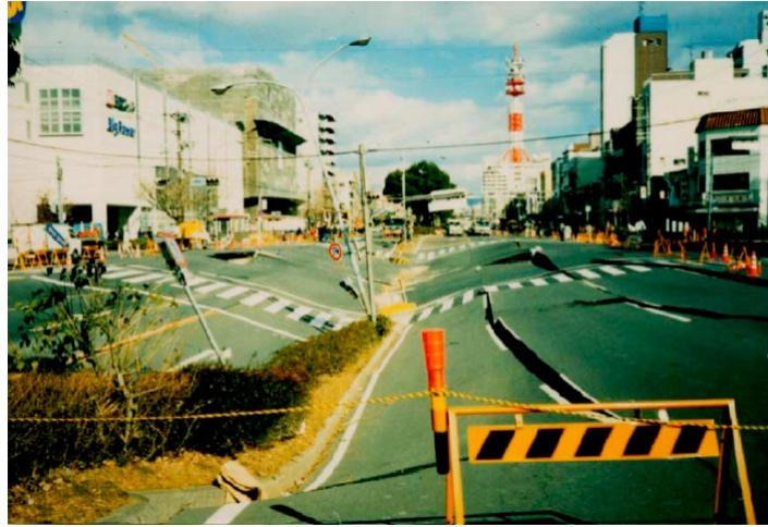
Figure 2. Severe deformation observed as a result of Daikai Station collapse (Uenishi and Sakurai, 2000)
