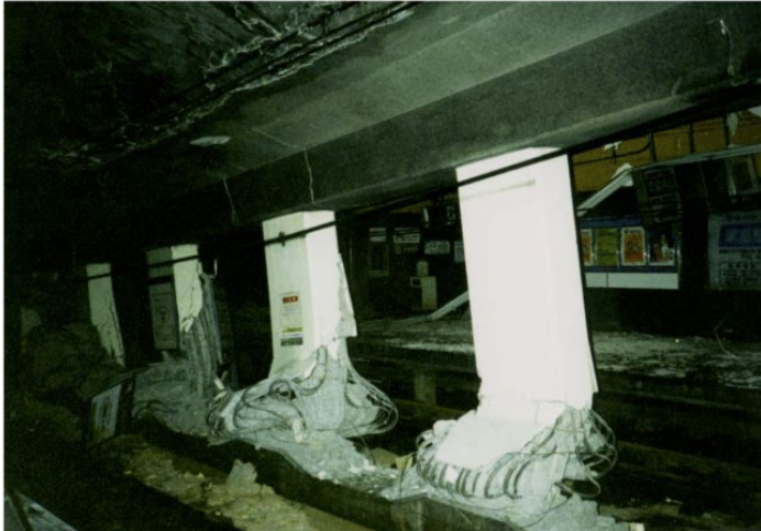
Figure 1. Damage to the central columns of Daikai Station (Uenishi and Sakurai, 2000)
