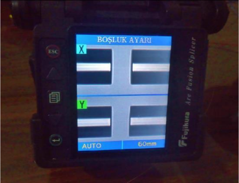
Figure 45. The utilized fusion splicer (Fujikura FSM 60S) to fuse two cables without signal loss
