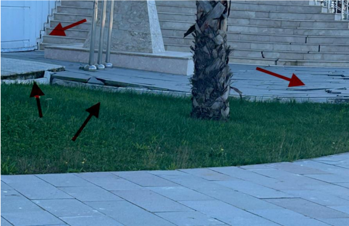
Figure 26. The surface deformations and cracks near the building
