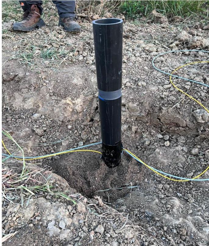
Figure 37. Appearance of an inclinometer pipe with two different fiber optic cables after placement in the monitoring site
