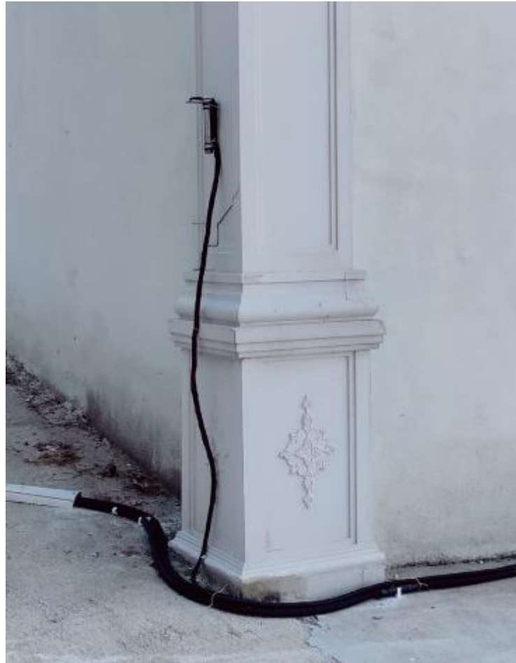
Figure 55. The strong ground motion station antenna is installed outside the data control room.
