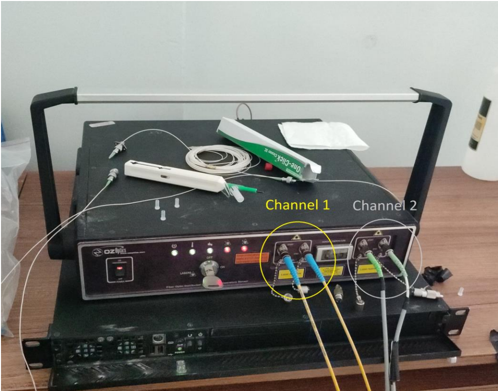
Figure 50. DSTS with two different fiber optical cables entrance and exit jacks
