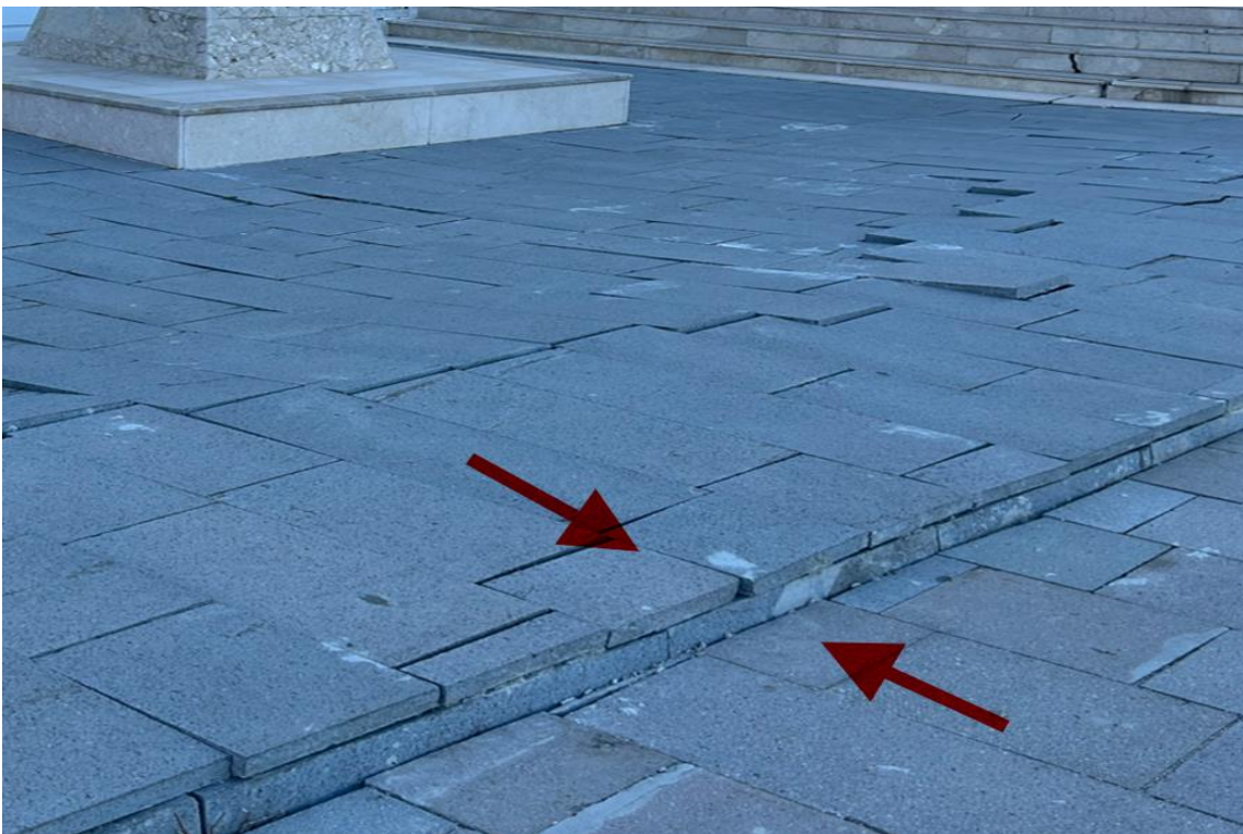
Figure 27. The surface deformations and cracks near the building
