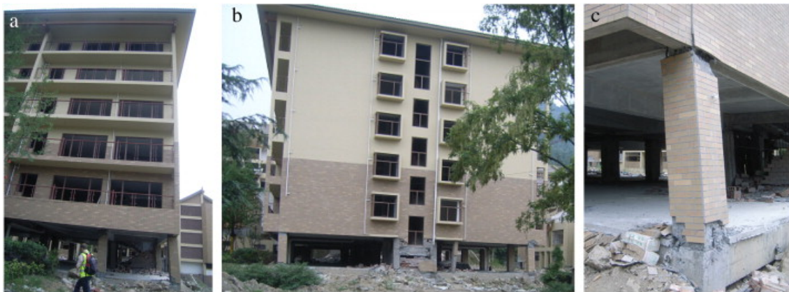
Figure 2.5 Formation of a Soft Story Mechanism After Wenchuan 2008 Earthquake[22]
