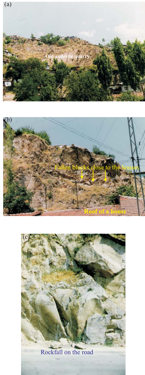
Fig. 2. (a) General view of the Timurlenk Hill and an old andesite quarry, (b) fallen blocks threatening a house, (c) rockfall on a road.
