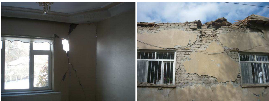
Figure 15. Improper placement of door and window openings
