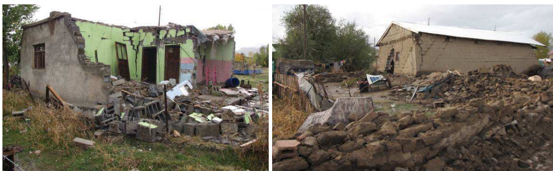
Figure 12. Improper mortar use such as mud
