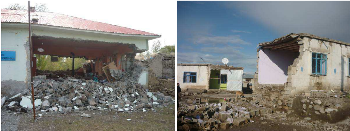
Figure 13. Poor wall-to-wall and wall-to-floor connections
