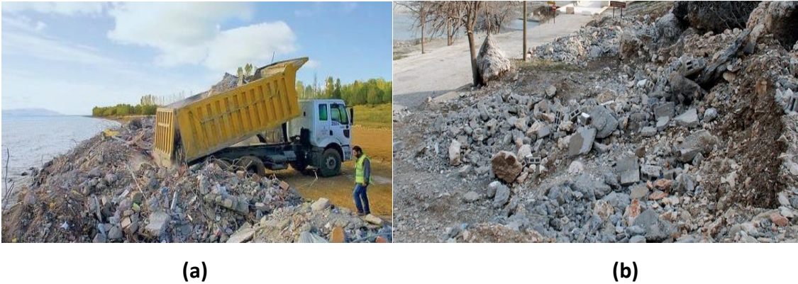
Figure 2. 7. Improper storage of (a) demolition waste, (b) rubble heaps
