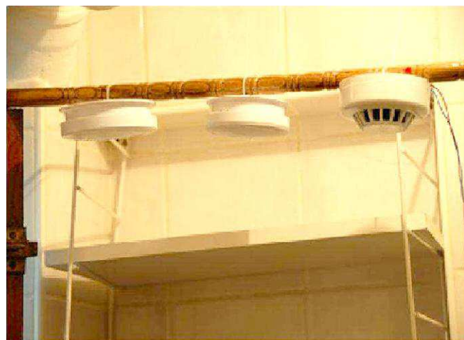
Fig. 9. Smoke sensors setup in a 4 m × 4 m small room with a ceiling height of 2.5 m.
