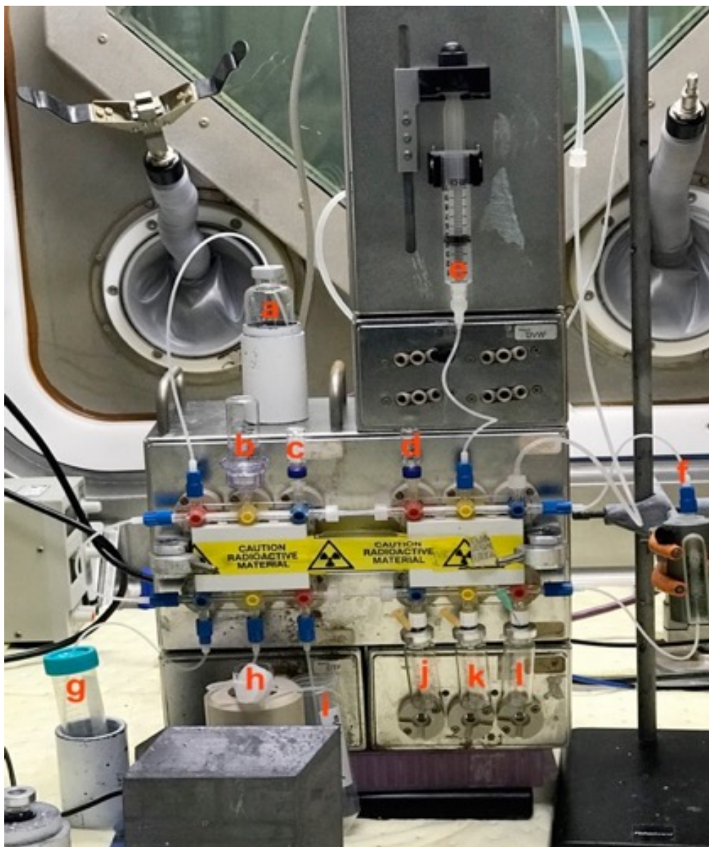
Figure 3.1. The cassette system which is used ^{89}\text{Zr} purification in hot cell.
